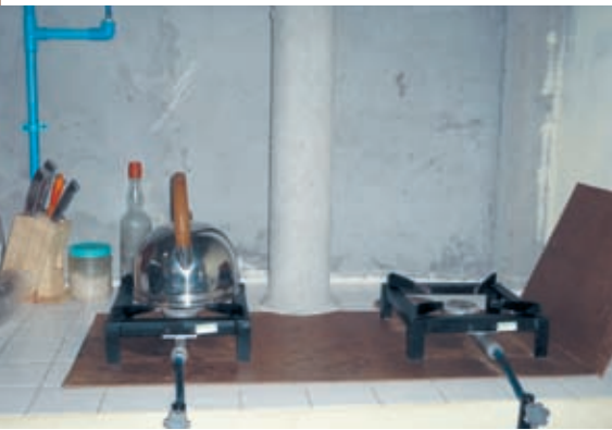
Farmer's kitchen with gas lines. The renewable energy is used here.
