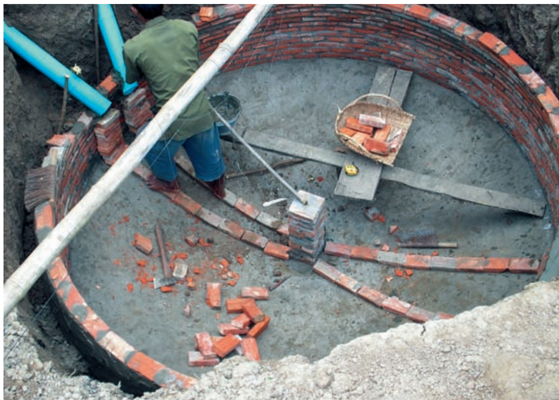
Laying PVC pipes: one to transport the manure, the other for excrement from the toilet.
