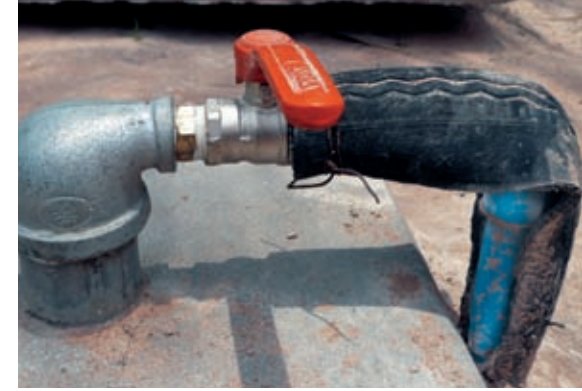
PVC pipes which transport biogas to the points of use are protected from the intensive rays of the sun by simple means such as old tyres.
